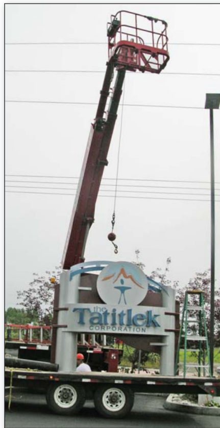
Super Signs installing the new sign at The Tatitlek Corp.'s new location using their crane truck, which can reach to heights of about 75 feet.
